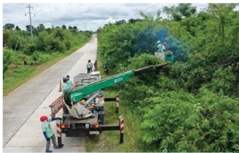
A total of 8.8 kilometers of electric line were cleared of obstructing trees/plants and vegetation during the line clearing activity.
