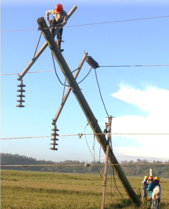
Rehabilitation of one (1) of a total of 98 downed structures of CAGELCO II's 69Kv Sub-transmission line.
