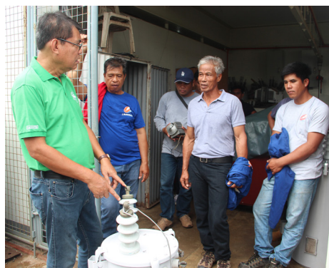
Engr. Felipe Radin, seminar's Resource Speaker, introduced the transformer polarity and voltage ratio test as part of the training.
