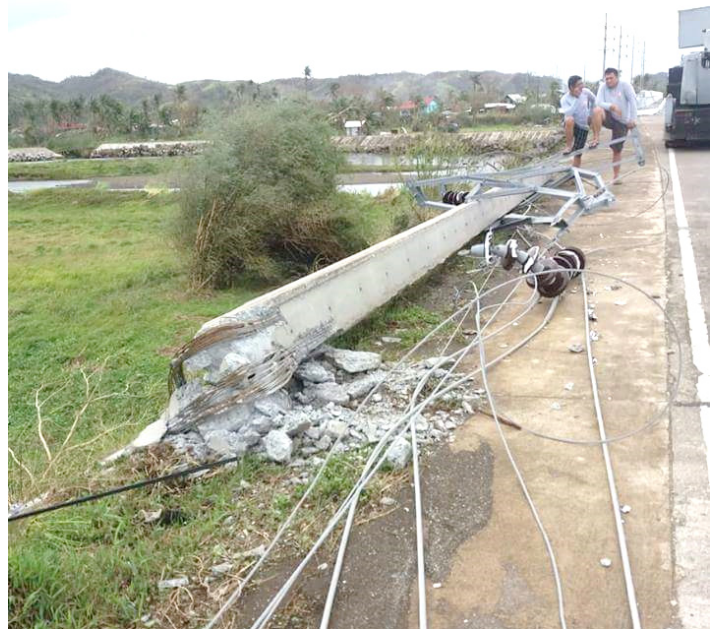
Broken concrete pole of 69KV Sub-transmission line at Sta. Ana, Cagayan.
